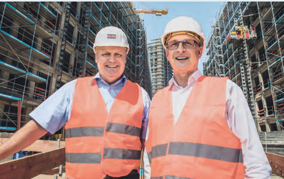
Markus Lentzler of ECE (right) and Jens Quade, subdivision manager at ZÜBLIN, regularly visit the MesseCity Köln construction site together.
