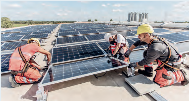
Installation of the pv system on the roof of the Mischek precasting plant
