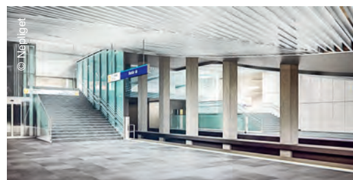
STRABAG is renovating the south section of the M3 metro line in Budapest
