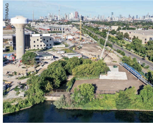
The pumping station will be built on this site of the Ashbridges Bay Wastewater Treatment Plant.
