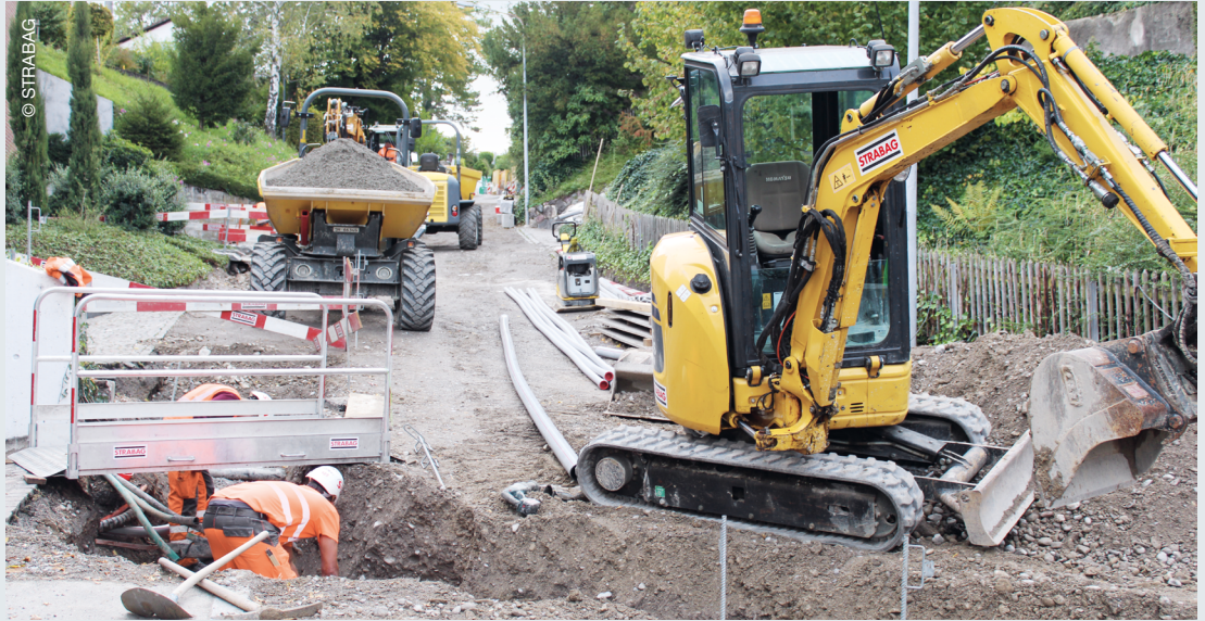
Construction work in Küsnacht (CH) with digitally accessible resident communication updated on a daily basis.
