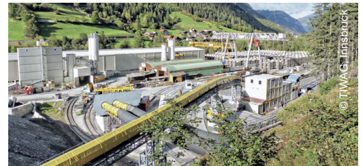
The run-of-the-river power plant on the Inn will make a significant contribution to Tyrol's energy autonomy.
