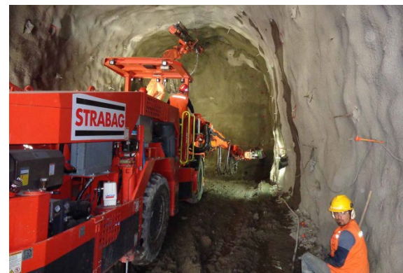
Alto Maipo power plant
