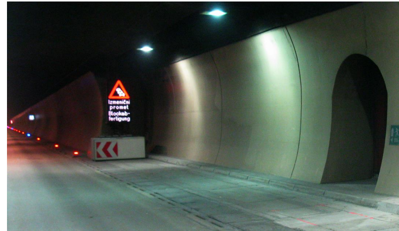
Tunnel technology and safety installations
