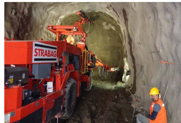
Alto Maipo power plant
