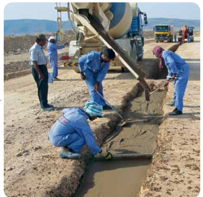
Pouring of the soil cement cutoff wall in the middle of the dam
