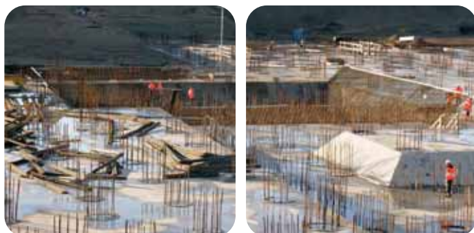
Foundation offset under the boiler house supports
