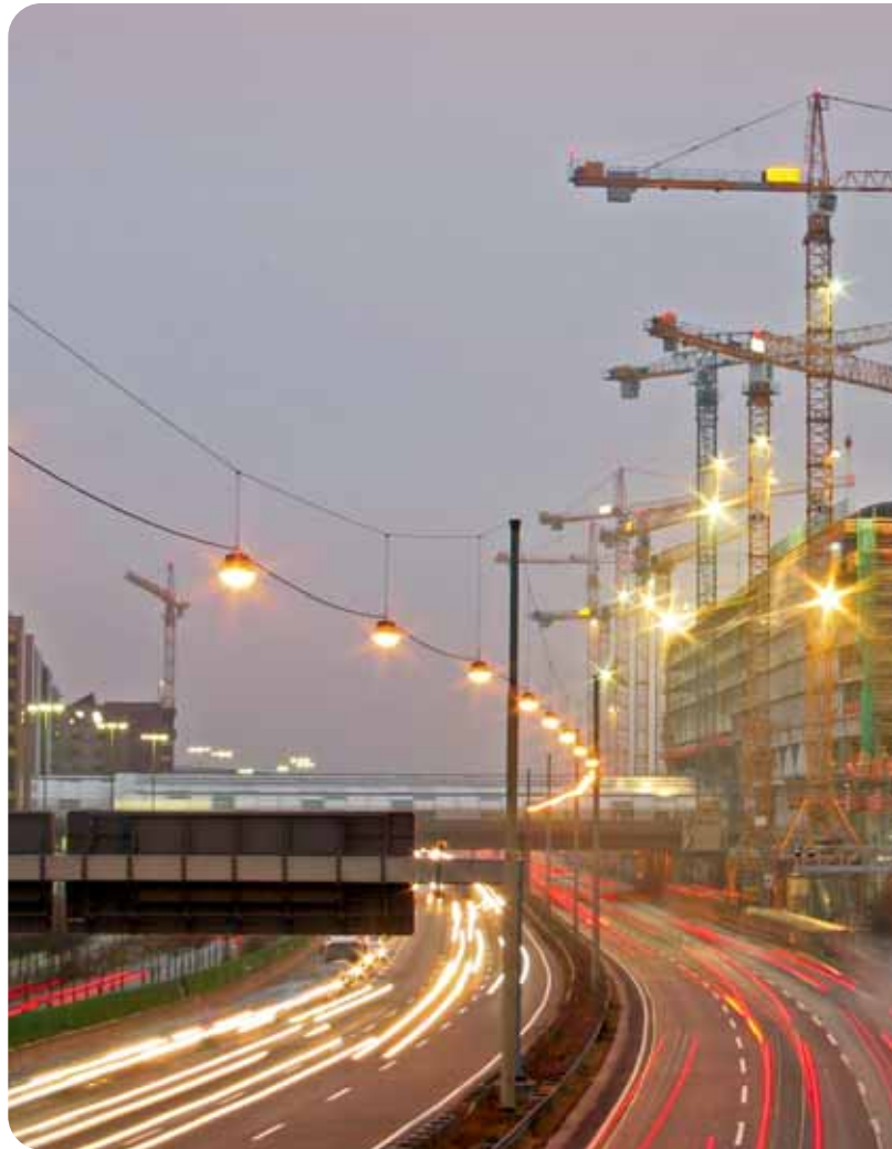
17 cranes in operation around the clock – the birth of the Airrail Center at Frankfurt Airport
