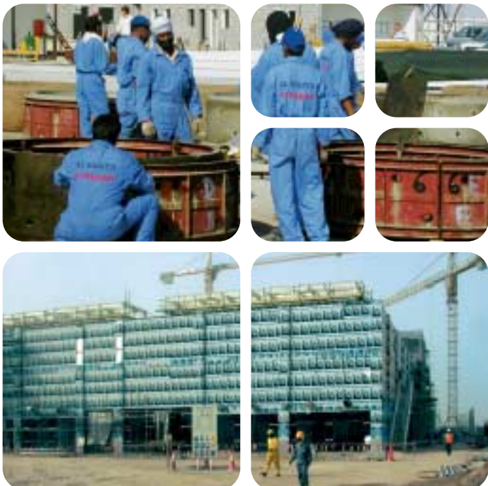
Top: Precast concrete element production for rain-water trenches in Wakrah. Bottom: The Injazat Data Center meets all security standards.
